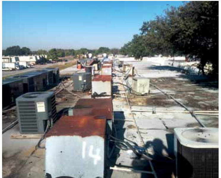
▲ New HVAC units for individual apartments and units yet to be replaced at CopperTree Apartments
