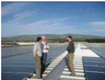
The PV array at SOMO
